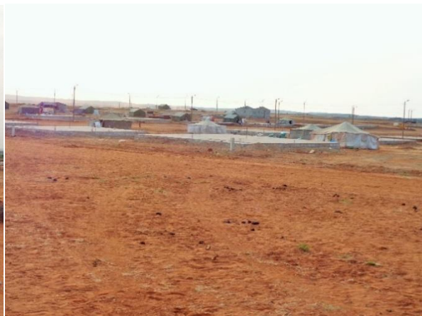
The foundations for the future homes at the Cabrais new settlement, August 2015.
